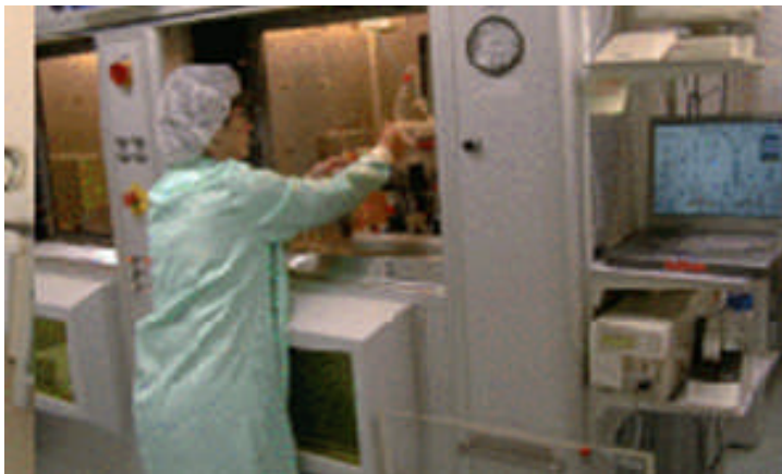
Hot cell & vault door interlocks, including fail safe interlock with automatic detection of probe failure.
