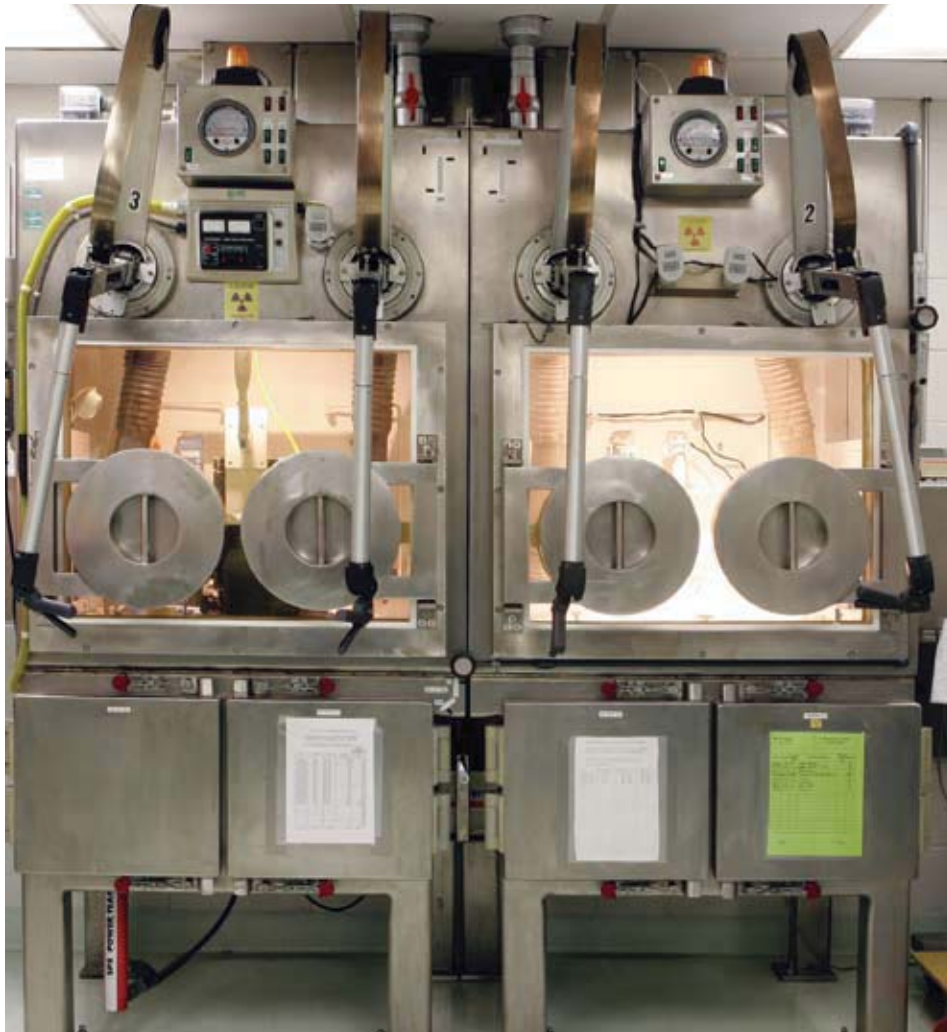
Eckert & Ziegler Isotope Products radiochemistry facilities used in the production of low-energy gamma sources.
